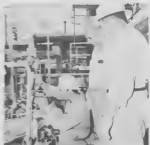
Overall view of new machinery at the Cat Naphtha Hydrofiner, Unit 22, on HDS site, shows Lago man at work.
